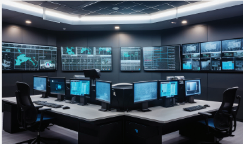
Control Room Display
